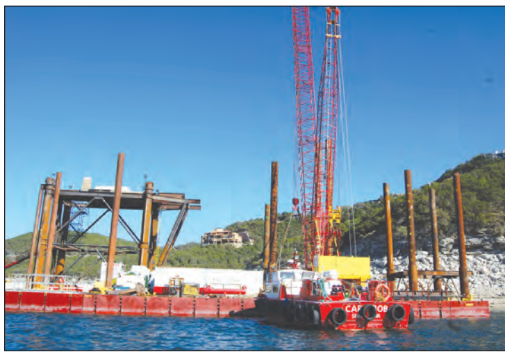
Four Points News staffer joined local media last week for a close-up view of the water intake phase of the City's new Water Treatment Plant #4. The structure is being built about three miles offshore from the system's staging site at Keller Marina.
