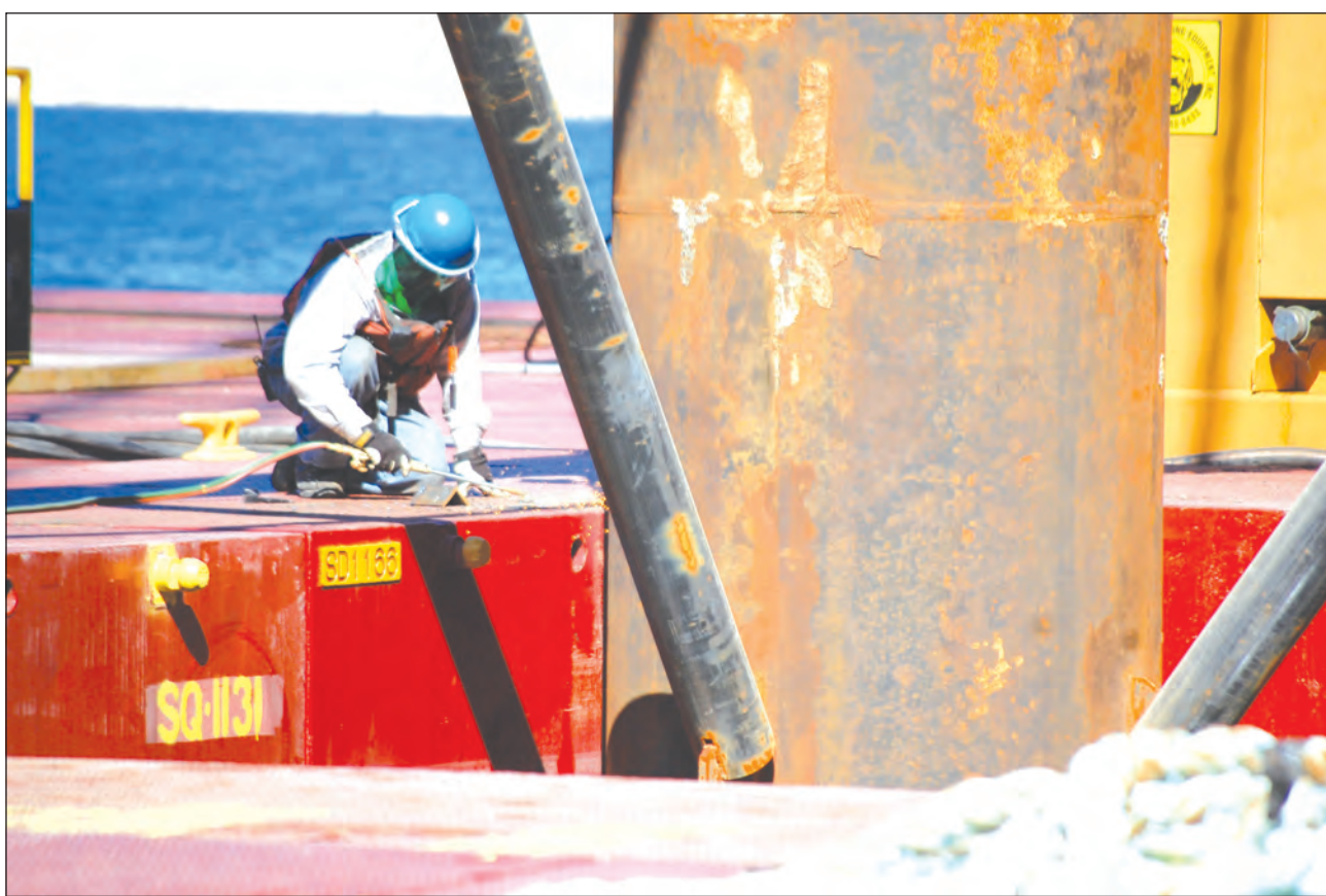
A welder works to construct one of three temporary platforms at the site of WTP4's raw water intake system on Lake Travis.
